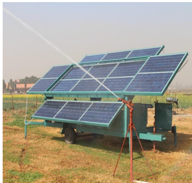
Figure 1: PSPS operating sprinkler irrigation system at National Agricultural research centre, Islamabad.
